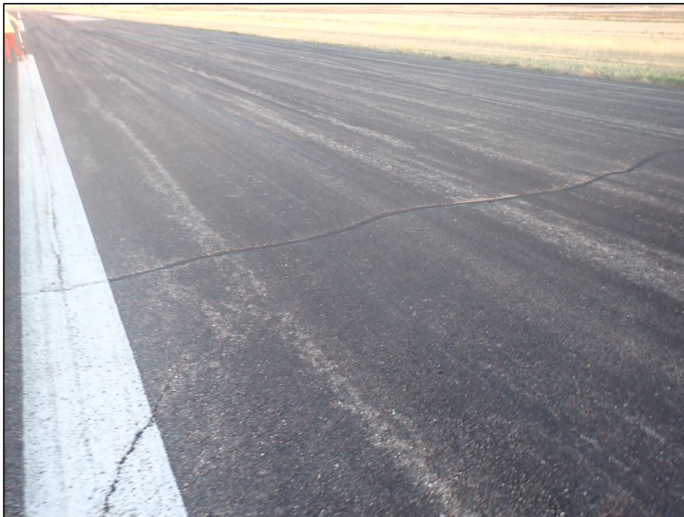
RW09-01-56: L&T Cracking
