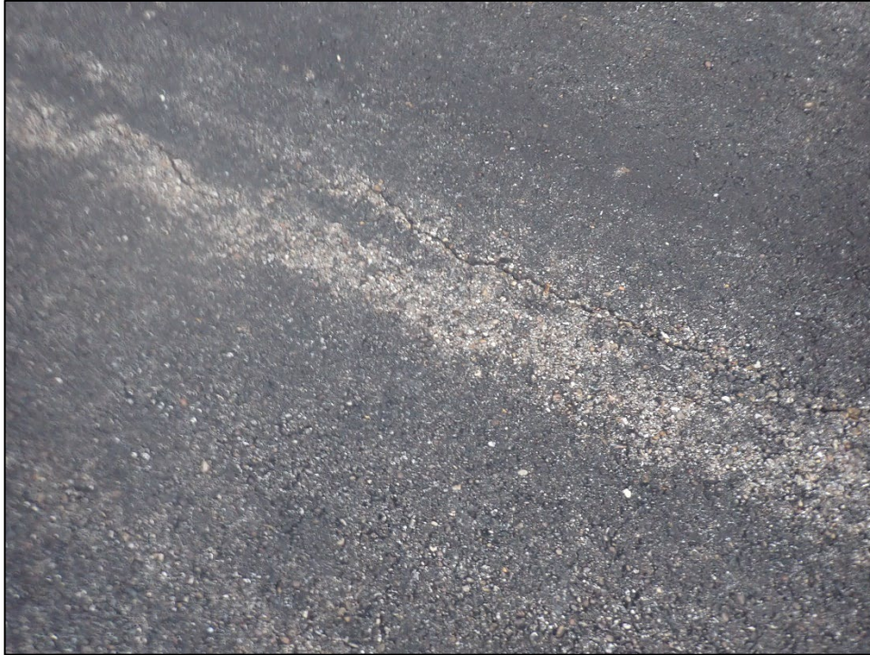
RW09-01-23: L&T Cracking
