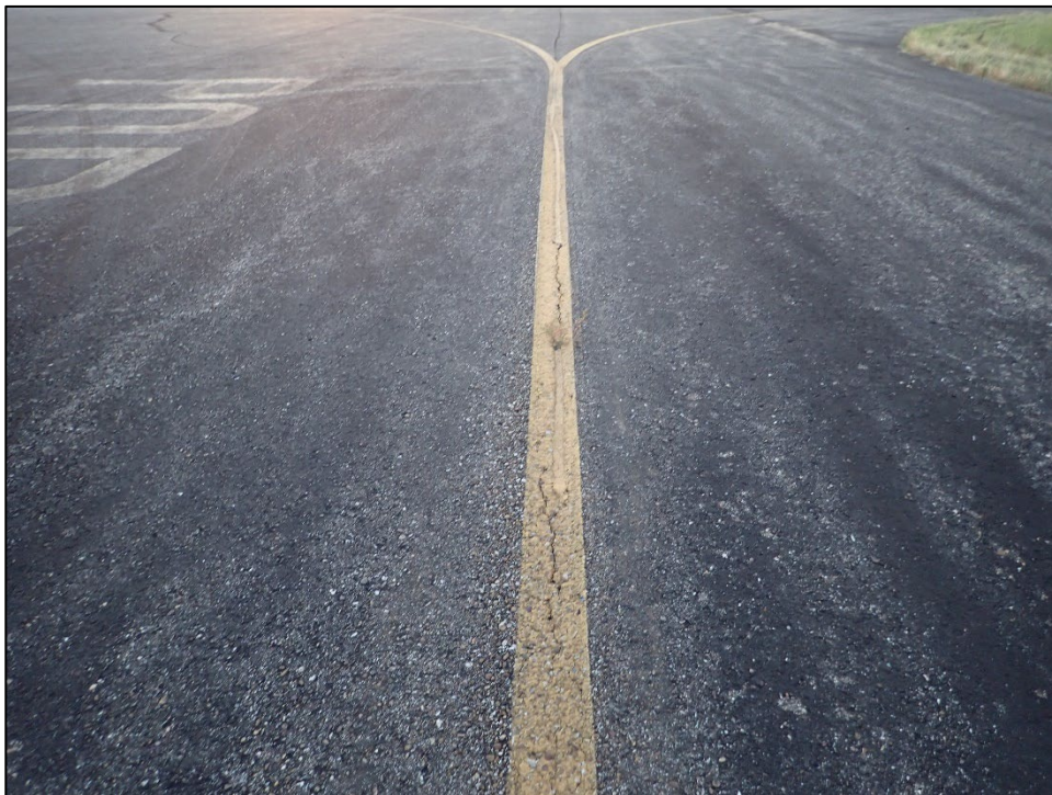
TW-01-11: L&T Cracking
